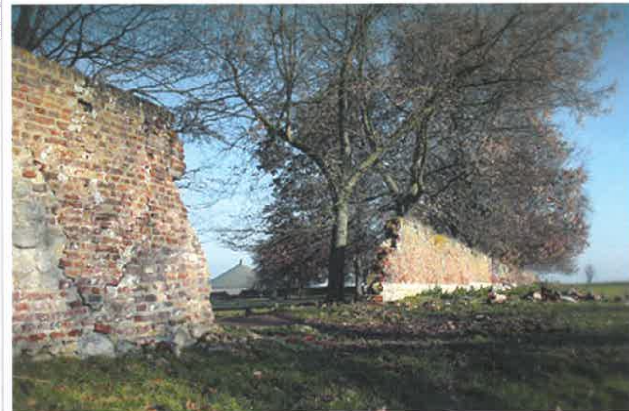
The Lion Mound seen through the hole in the southern wall of what was Hougoumont's Formal Garden
